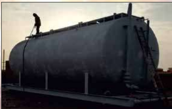
500 BBL Skid Mounted Storage Tanks
