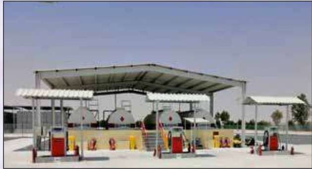
Fuel Station ADNOC Labour Camp Habshan
