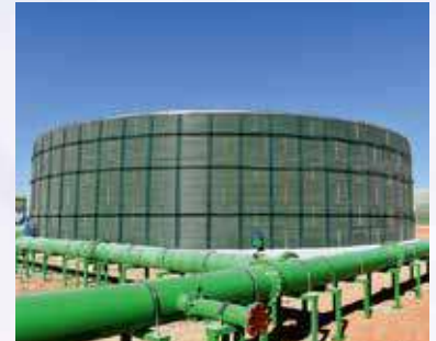
Bulk Water Storage Tanks
